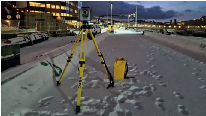
▲ Work on the Bergen Light Rail Project is not delayed by winter weather. The Trimble SX12 operates in the cold without issues. (Courtesy: NCC)
