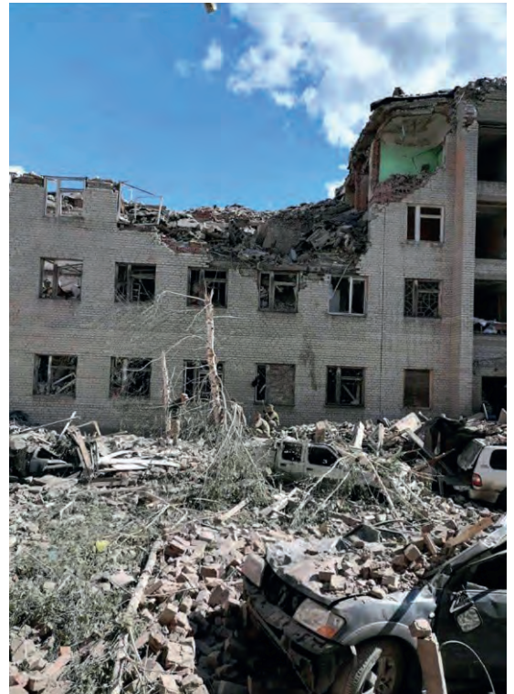
▲ 50 premises are presently totally unavailable, such as the destroyed regional office in Bahmyt. (Image courtesy: StateGeoCadastré)
