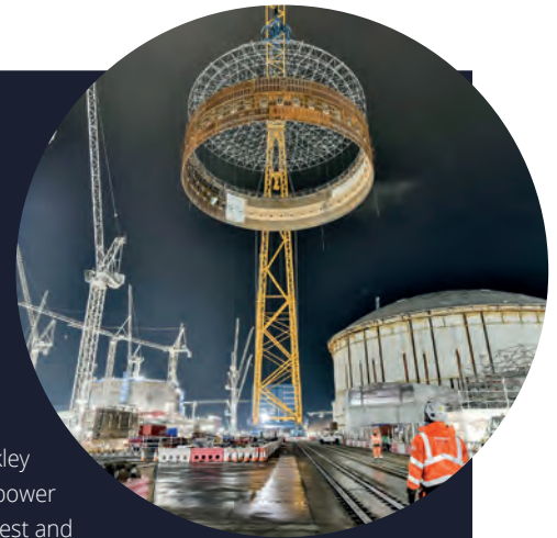
▲ Big Carl, the world's strongest land-based crane, looms over Hinkley Point C nuclear power station. It is capable of hoisting a staggering 5,000 tonnes in a single lift. (Image courtesy: EDF)
